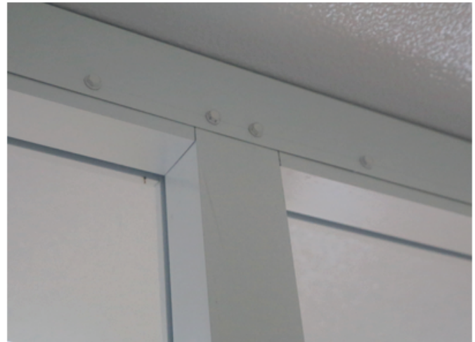
2x2 Mainframe in Top Uchannel ( with 1x2 installed)
